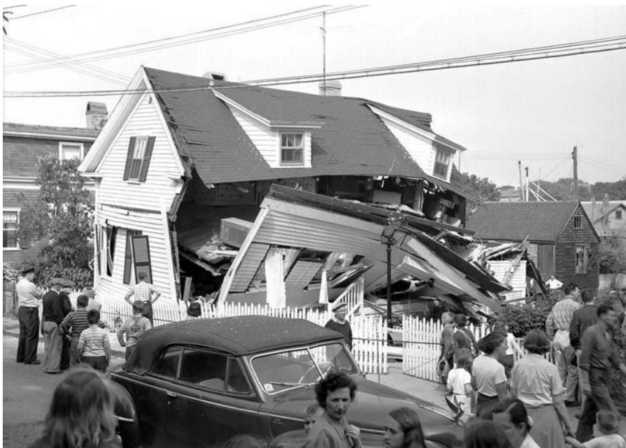
25 Orne Street following a gas explosion on June 4, 1951. (Courtesy of Dan Dixey's Marblehead Historic Images)
